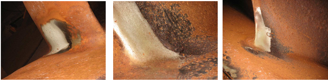
Fig. 1- Hydraulic turbine blades damaged by cavitation and crack repairing.
