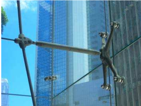
Fig. 1: Structural application of tempered glass (Point fixed glass in-plane loaded, 3 Pacific Place, Hong Kong)
