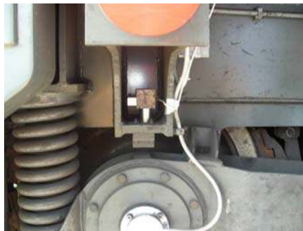
Fig. 10 The position of the acceleration on the carrier of the bogie, above the axial assembly
