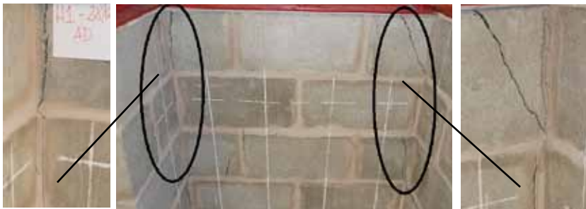
Figure 9 — Failure mode of specimen.
