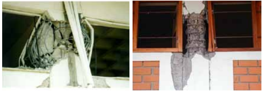
Figure 1 — Examples of short column failure: a) 5-story building, built in 1997 according to the new Greek Seismic Code, [2]; b) Ø10 mm at 10 cm transverse reinforcement did not prevent heavy damage, [3]
