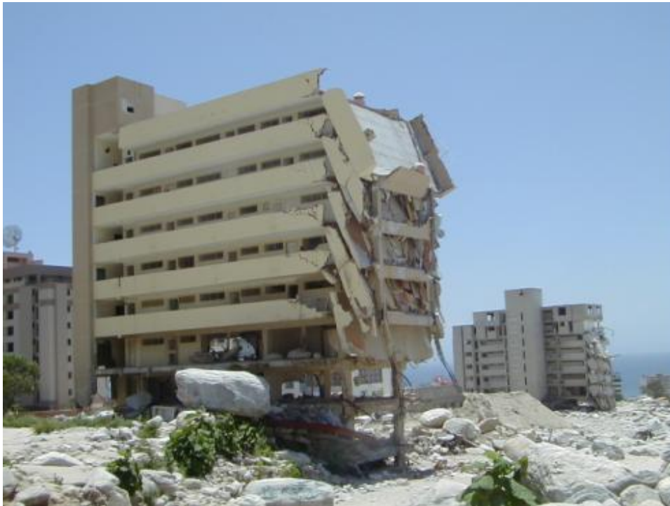
Figure 1.2-9 damaged by passage of debris-flow from (Wieczorek, Larsen, Eaton, Morgan, & Blair, 2016)
