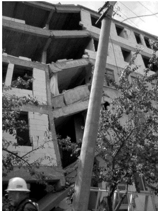
Figure 1.2-6 Multi-story building intersected by faulting from (Scawthorn & Johnson, 2000)
