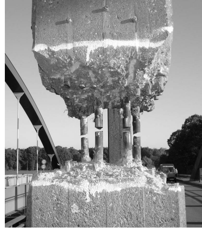
(b) Severed Hanger
