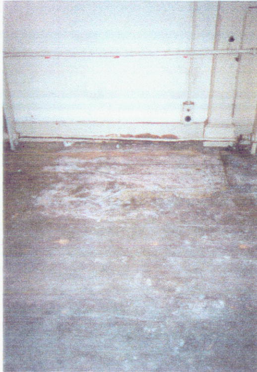
Figure 5.6 : Colony extent and floor damage six months from start of experiment.
