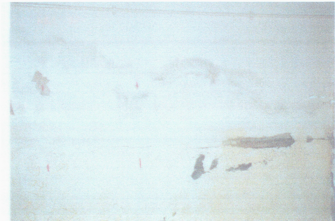
Figure 5.15 : Water damage to the plaster above the fireplace. Note the presence of moulds at the leading edge of the water damage.
