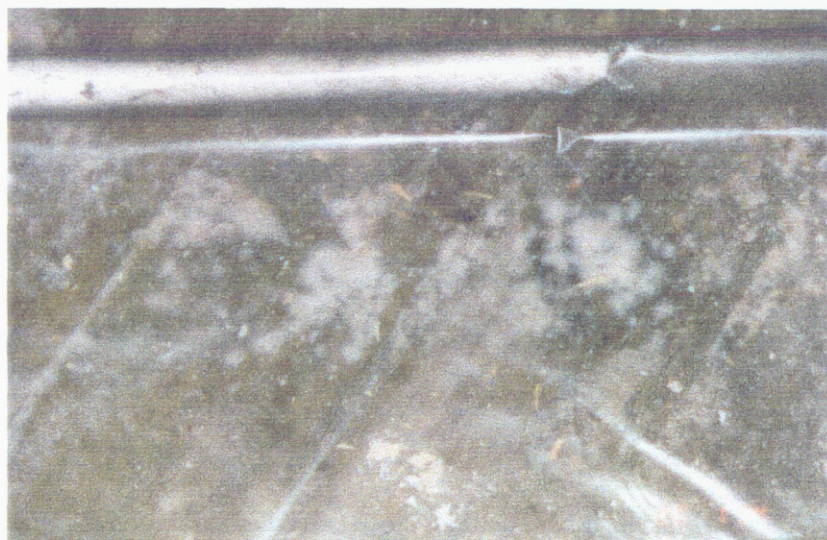
Figure 5.7 : Growth of S.lacrymans under the plastic sheeting. Note formation of moisture on the underside of the sheet.
