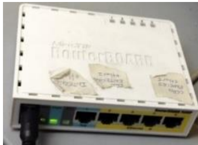
Figura 3.4: Router Board - Mikrotik 750 up.
