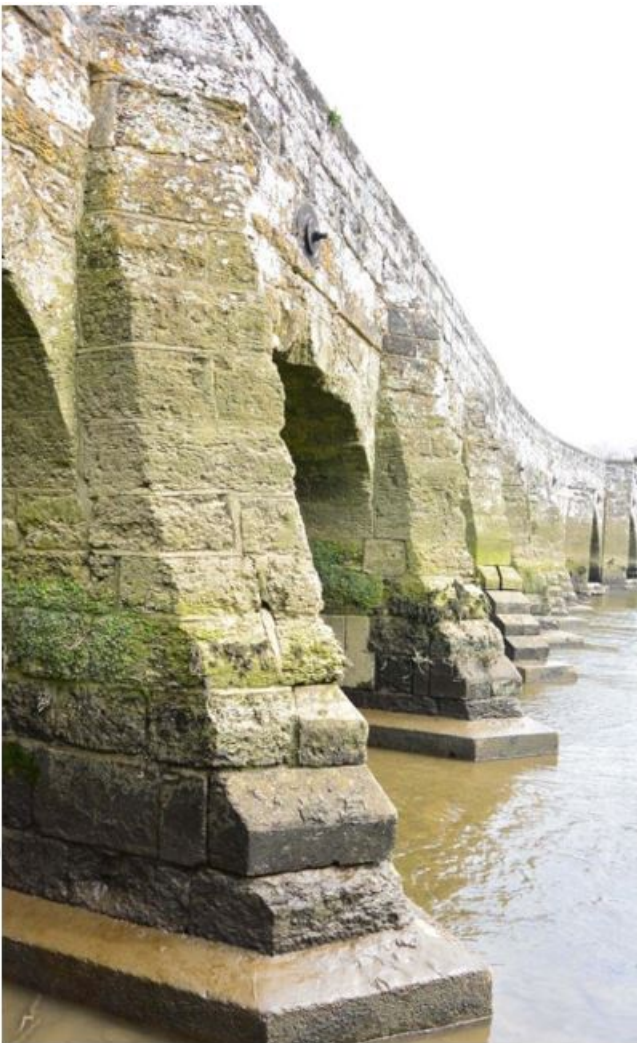
Fig 14 Eroded stone work prior to 2018 refurbishment
