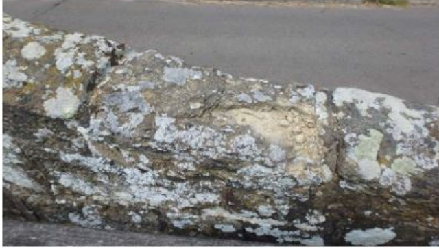
Fig 13 Eroded stone work prior to 2018 refurbishment
