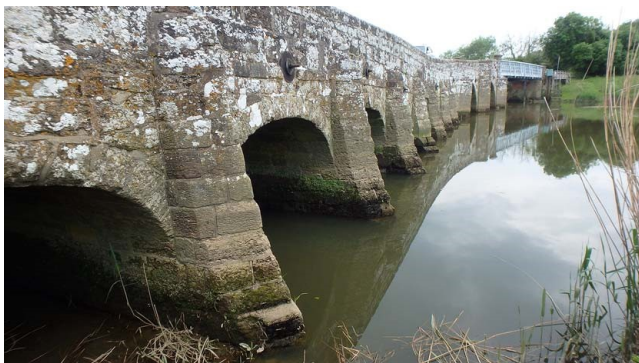
Fig 12 Eroded stone work prior to 2018 refurbishment
