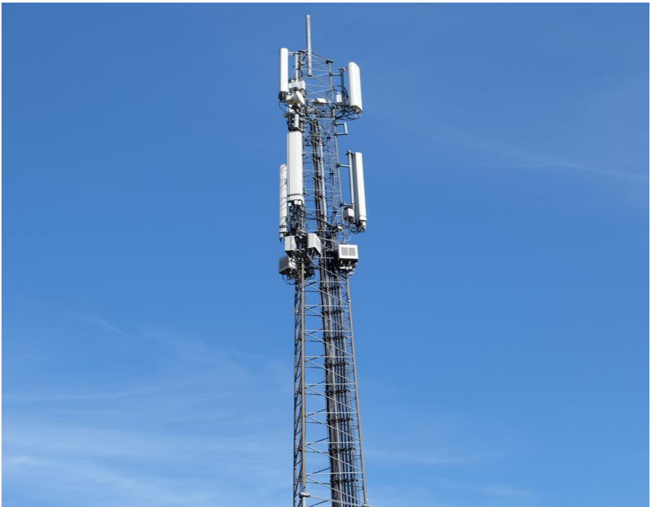
Figure 8. A base station with antennae attached to a tower.
