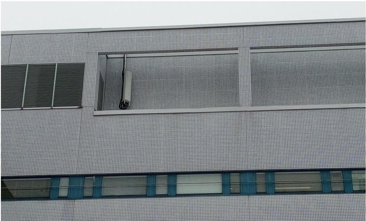
Figure 7. A base station antenna mounted on the side of a building.
