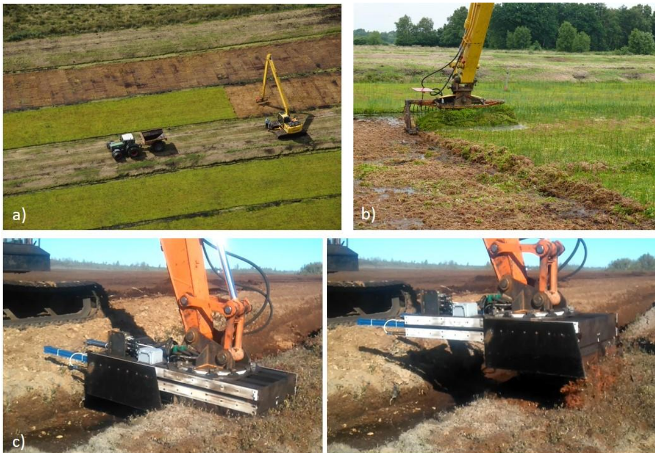
Figure 7. Harvesting techniques for Sphagnum farming using a) an excavator operating from a causeway, equipped with b) a mowing bucket or c) a modified excavator for block-cut peat extraction, which tests in Canada have shown can also harvest Sphagnum . Photos: a) Gerd Block, b) Sabine Wichmann and c) Benoit St-Hilaire).
