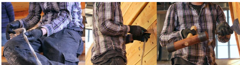
Figure 8. Traditional caulking process: preparing oakum (left); putting oakum into the seams with a sleek (centre); pressing oakum with a caulking iron and caulking mallet to seal the seam.
