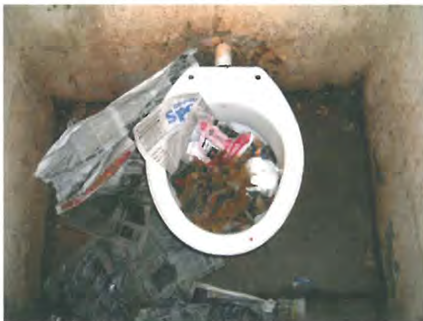
Plate 3.2: Blocked communal toilet in Duncan Village still being used by residents
