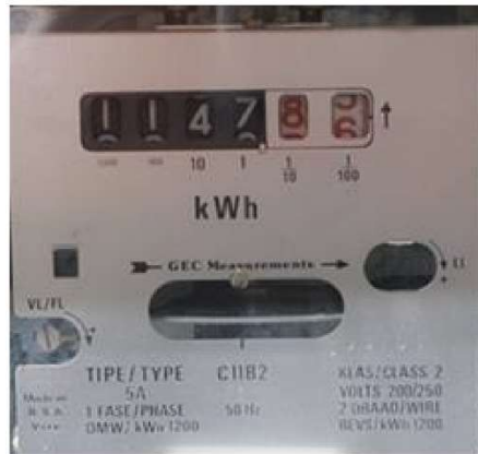
Figure 6: Electricity meter with kWh output (Zietsman, 2015)
