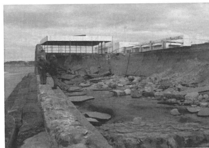
Figure 7. Destruction of Punta Candor protruding paved area after the storm of December 2004.
