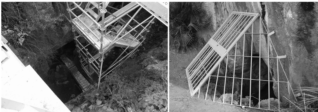
Fig. 4. Security structure in the entrance of the karst complex and closing of the “Sima”.
