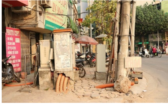
(b) Electric station in sidewalk in Hanoi
