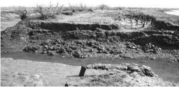
Photo 1 : Brèche de Graveyron à marée descendante, mars 2004 (cl. C. Marcadet) The breach of Graveyron during falling tide, march 2004
