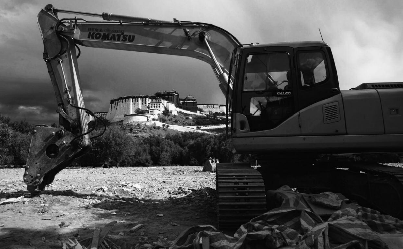
A grab parks at a construction site behind the Potala Palace on 27 June 2006 in Lhasa, Tibet Autonomous Region, China. © AFP
