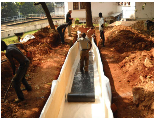
Figure 1b. Installing the filtration materials: 4-8mm and 0-4mm sand separated from 20mm aggregate by geotextile
