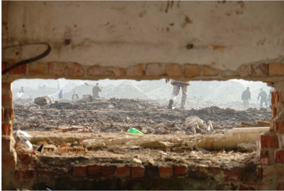
Figure 1 - The wall of a XIX th century factory, after demolition. Credits: Liviu Chelcea.
