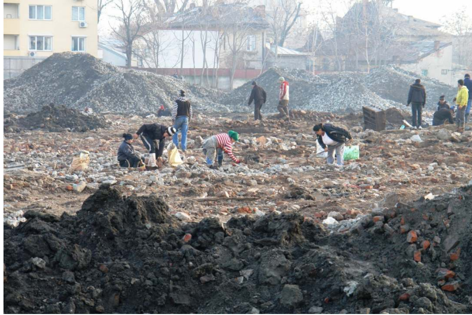
Figure 2 - The yard of the same demolished factory (Timpuri Noi), a couple of days after its demolition. The owner allowed about 50 to 100 people to enter the premises, dig for the scrap metal and carry it to a collection center situated about 150 meters away. Credits: Liviu Chelcea.
