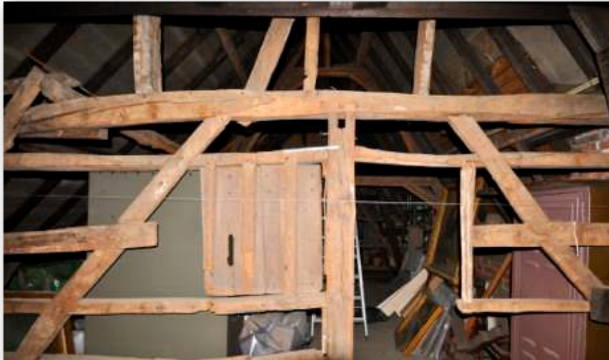
Fig. 3: Anderlecht Beguinage, 8 Rue du Chapelain. View of the attic of the west building of the complex, built with bricks in the 17th century. In the foreground, the roof truss n° 2 is a structure built from the former facade truss of a mediaeval half-timber building perhaps dating from the 18th or 19th century (© Paulo Charruadas and Philippe Sosnowska, Centre de Recherche en Archéologie et Patrimoine, Université Libre de Bruxelles, 2010)
