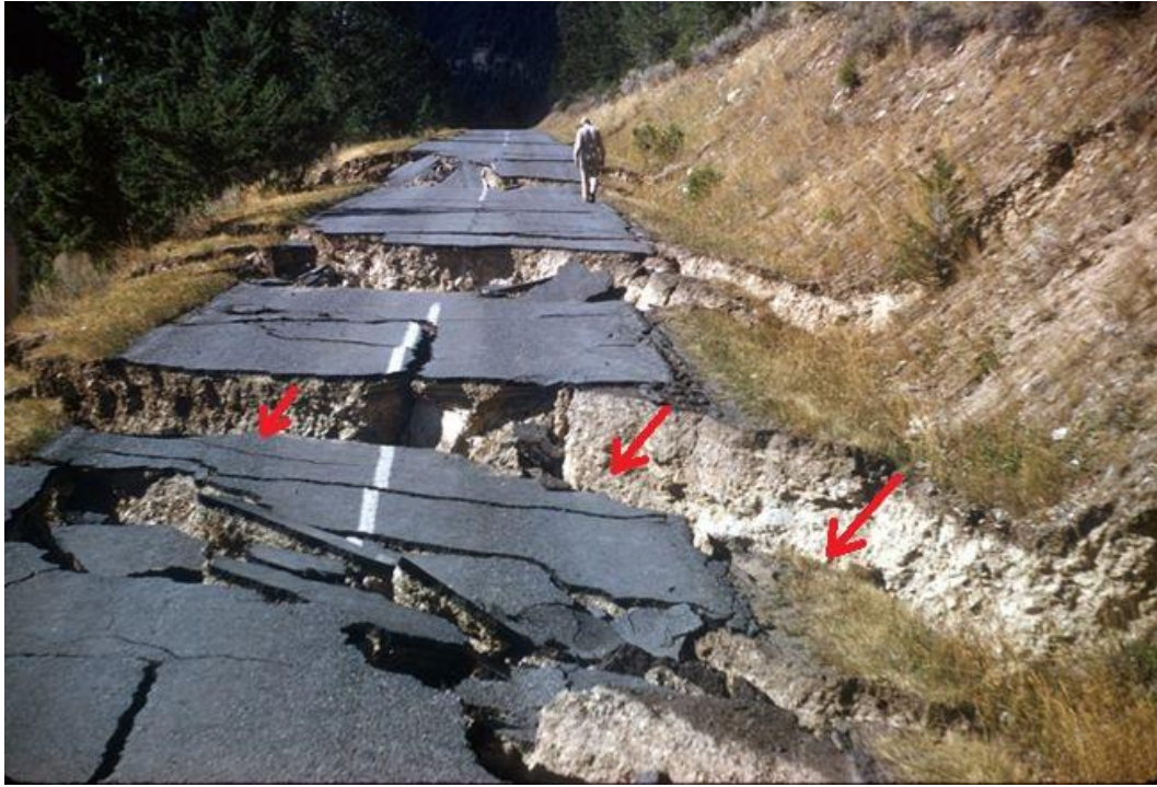
Figure 1.4 Lateral spreads at Hebgen Lake near West Yellowstone, USA. Shaking from the M_w=7.2 August 18, 1959, earthquake. The red arrows depict the main directions of motion [Adapted from USGS].
