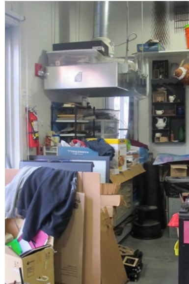
Figure 4.11.2. Site 11 blocked ventilation hood.
