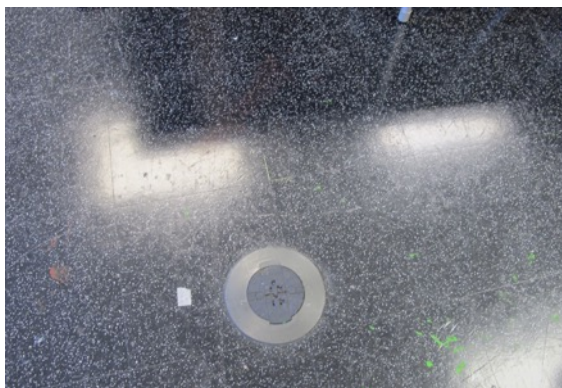
Figure 4.4.21. Site 3 floor embedded electrical outlet.
