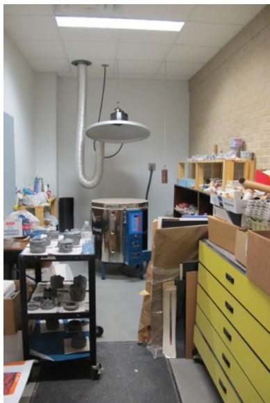
Figure 4.10.3. Site 5 storage room equipped for kiln uses.
