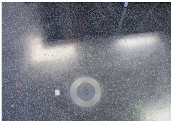
Figure 4.7.5. Site 3 floor-based electrical outlets.
