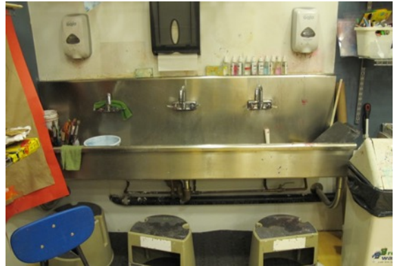
Figure 4.2.2. Site 7 ADA compliant sink?
