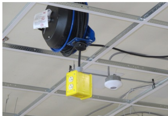
Figure 4.4.22. Site 18 ceiling mounted electrical outlet.
