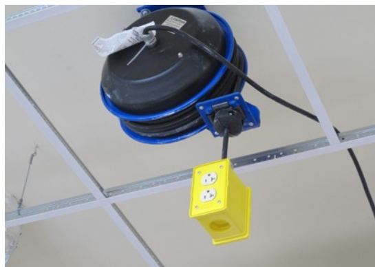
Figure 4.7.6. Site 18 ceiling mounted electrical box.
