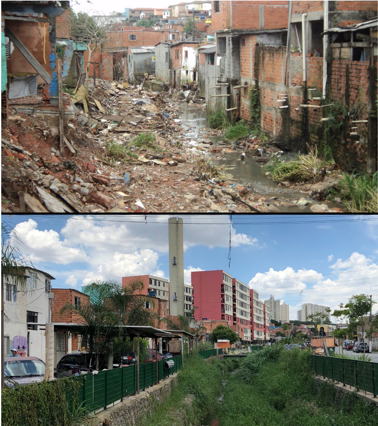
Figure 9. Sapé creek before upgrading (above) and after the works (below). Sources: SEHAB and the author.
