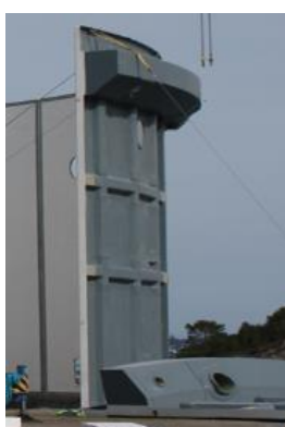
Figure 3-4. Detail from picture of Aquafarm CCS under construction possibly showing integrated GRP buoyancy ring
