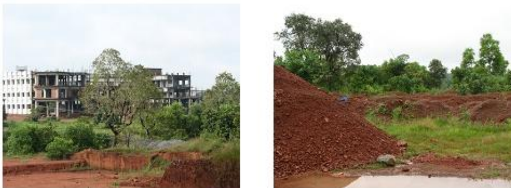
Fig4.3: Recent site disturbances: a) View of the engineering college building on Nasrāṇikunn from an adjacent hill . b) Debris accumulated on the north western part of Nasrāṇikunn due to recent construction activity (photos: Author 2010)
