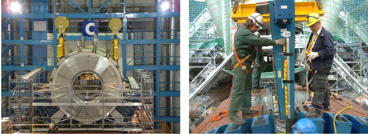
Figure 21. Installation of the barrel cryostat in the ATLAS cavern (left). The installation of the final TileCal module in the EBC calorimeter (right).
