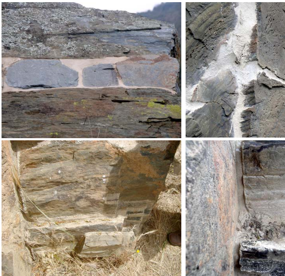
Figure 3 - Aspects of solutions proposed by the contractors. Bridging a large gap to avoid excessive water infiltration (upper left); details of the mortar filling of wide fracture gaps (upper right and lower left) and detail of the filled gap after a flooding episode (lower right).
