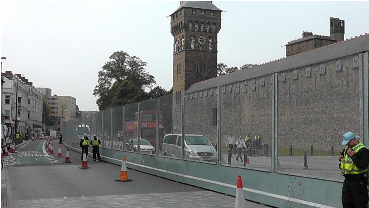
Picture 48: Street View of Steel Perimeter Fence Installed to Protect the Walls of Cardiff Castle
