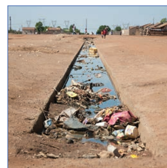
Clogged drain, Zambia
