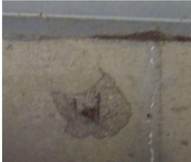
Figure 54: Zoomed-in view of part of the underside GoPro image featuring a spill that was visible using the waterproof UAV, without having to send a person under the bridge.
