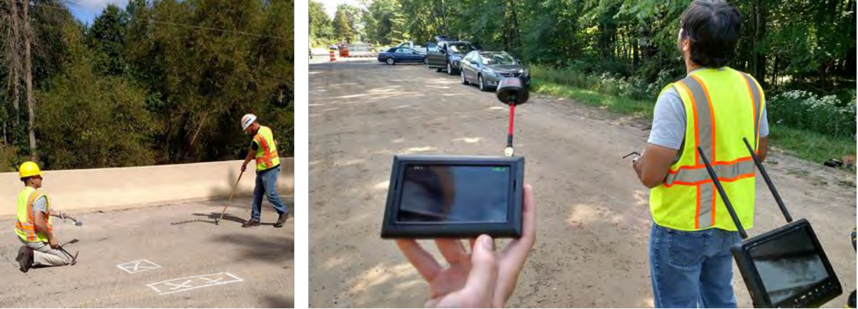
Figure 3: Gordonville Road data collection photos: MDOT staff collect ground truth delamination data with chain dragging (left); R. Dobson collects thermal data with the Bergen hexacopter and FLIR Vue Pro combination with real-time display of the thermal data visible in two first-person viewer screens (right).
