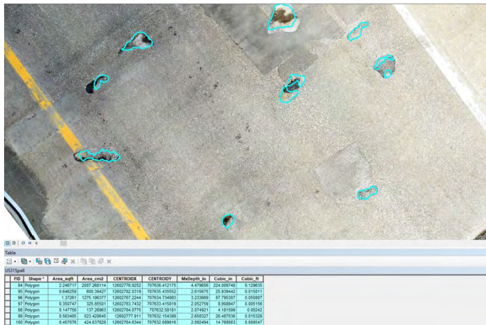
Figure 94: Example output from the Spalgorithm tool from the US31 bridge dataset showing detected spalls and associated attribute data such as area and maximum depth.
