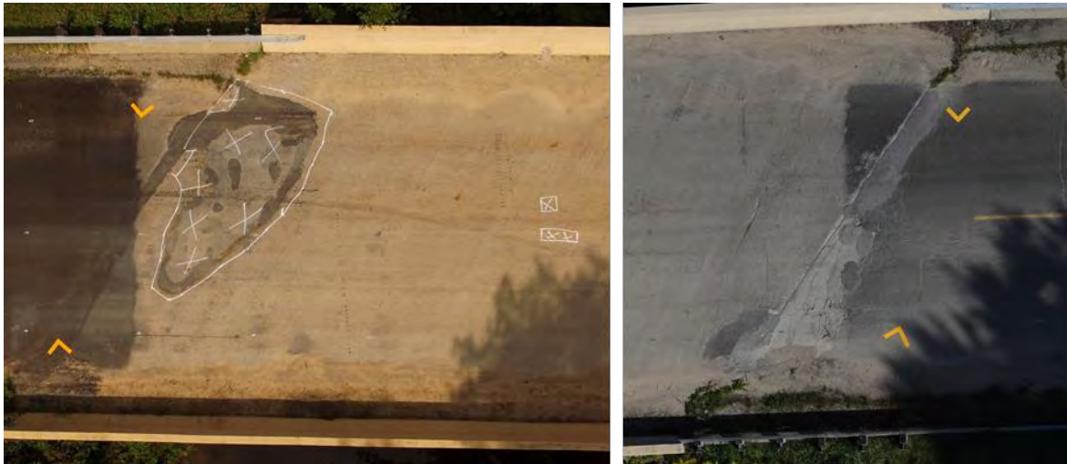
Figure 4: Example digital camera images from the Gordonville Road site: a DJI Phantom 3A image showing surface patching and sounding survey markings (left); a Nikon D810 image showing part of the bridge with distresses at the eastern bridge joint. Both photos have GPS ground control markers visible (yellow chevrons).
