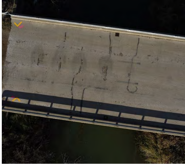
Figure 10: Nikon D810 image of the Uncle Henry Road bridge deck.
