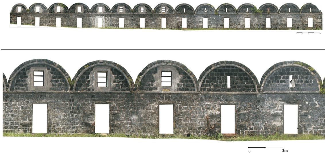
Fig. 3 Trianon barracks. Upper: photogrammetric representation of the entire row of barracks; lower detail of individual barracks
