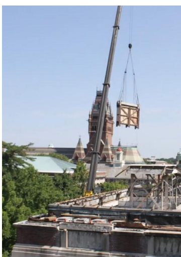
Moving Hunger March via crane onto an air-ride flat-bed truck for transport
