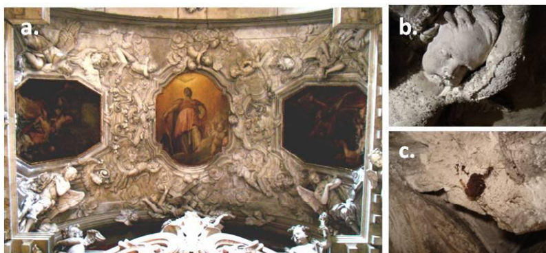
Fig. 1 (a) Vault of the Addolorata Chapel in San Pantalon's Church; (b) material losses and spalling (c) detachment and rusty iron rods
