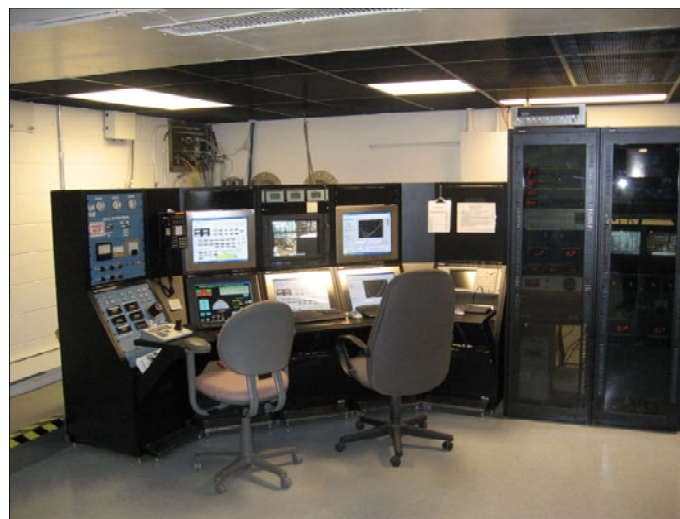
Figure 7. Acoustic Research Tunnel Control Room.
