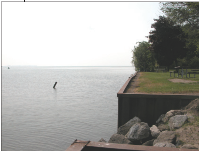
Figure 1. Lake Erie shoreline hardening with steel sheet piling (Photo credit: Greg Norwood).
