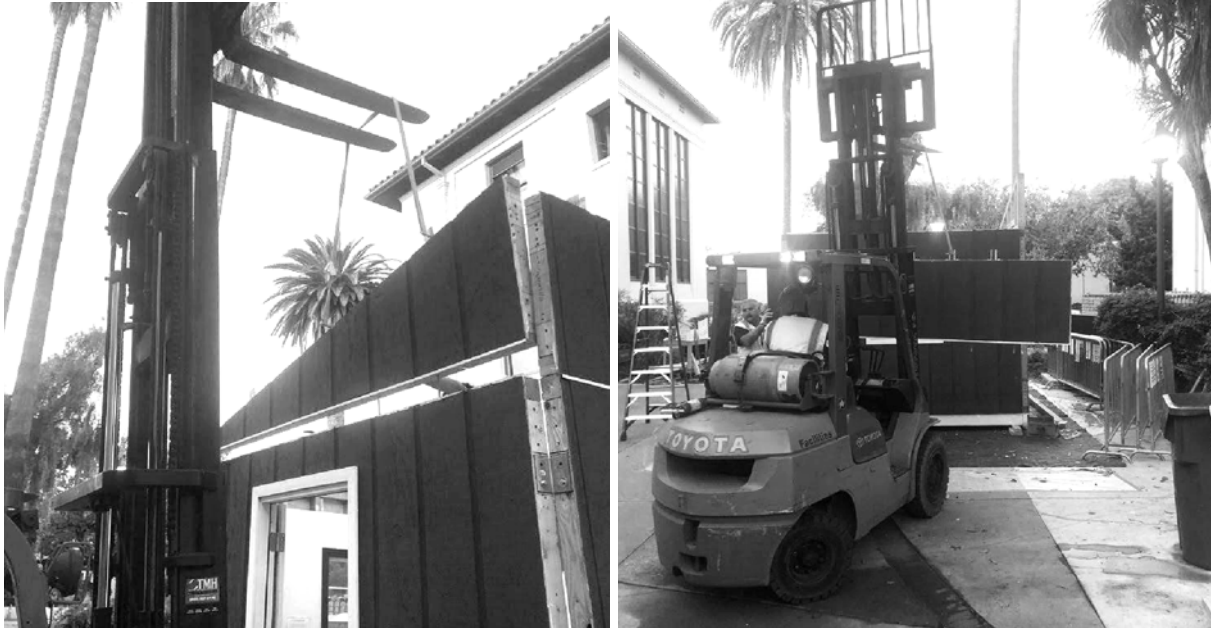
Figure H.17 - The height extensions were removed by connecting straps to the A24 brackets on top of the extensions.
