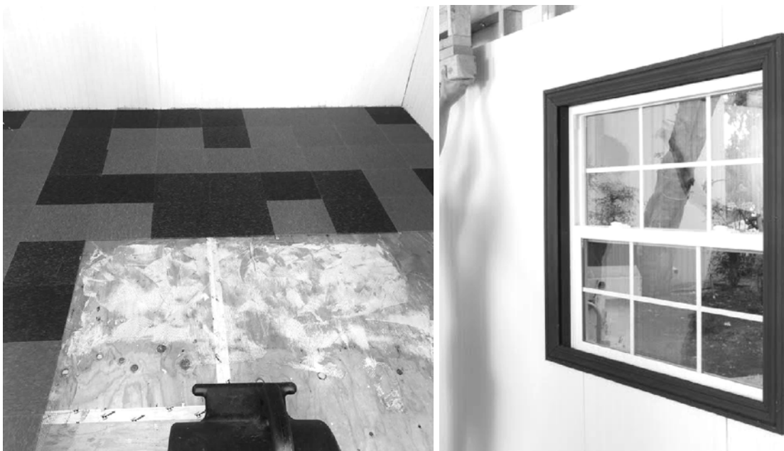
Figure H.14 - The vinyl flooring was installed on the plywood subfloor (left) and interior trim was installed (right).
