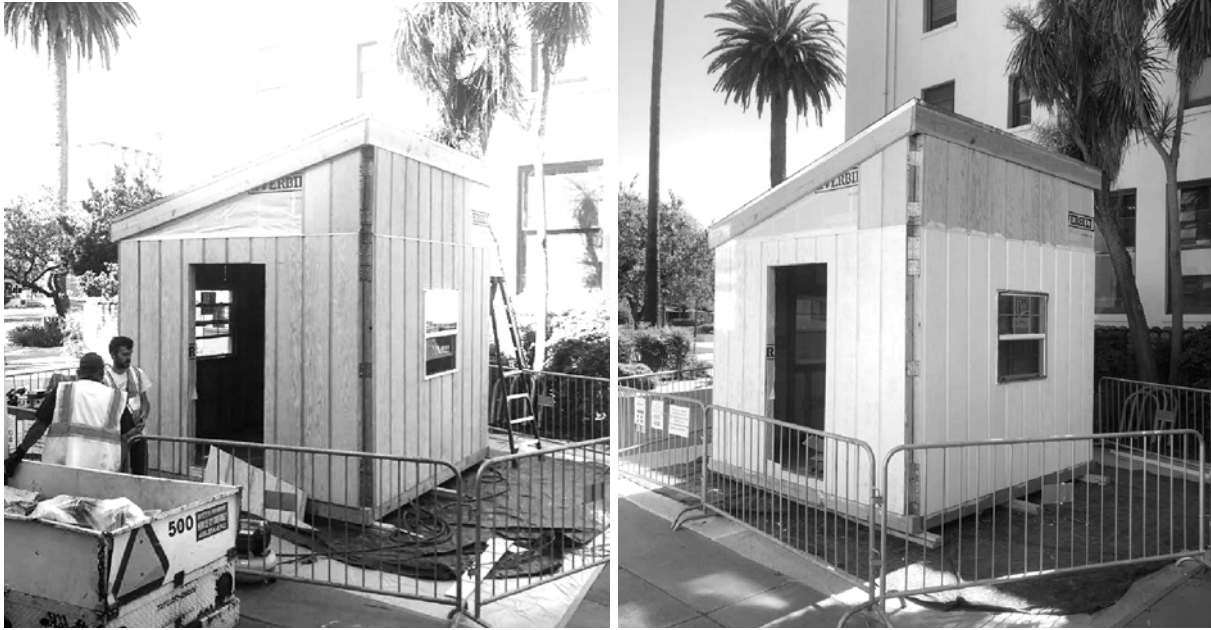
Figure H.11 - The exterior sheathing was installed (left) and primed for paint (right).
