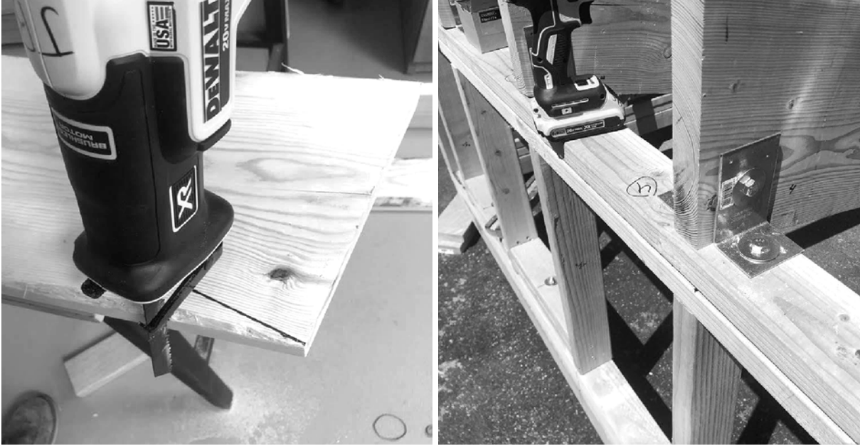
Figure H.7 - The roof joists were cut (left) and the roof was framed on the height extensions (right).
