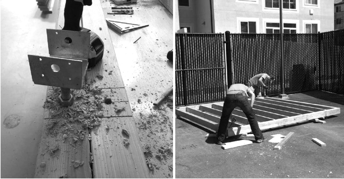
Figure H.3 - The floor beams were prepared for the wall-to-floor connections (left) and then the floor was framed (right).
