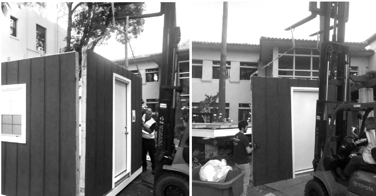
Figure H.18 - The walls were removed and carried using straps wrapped around bolts connected into the T-nuts used for the wall-to-wall corner connections..
