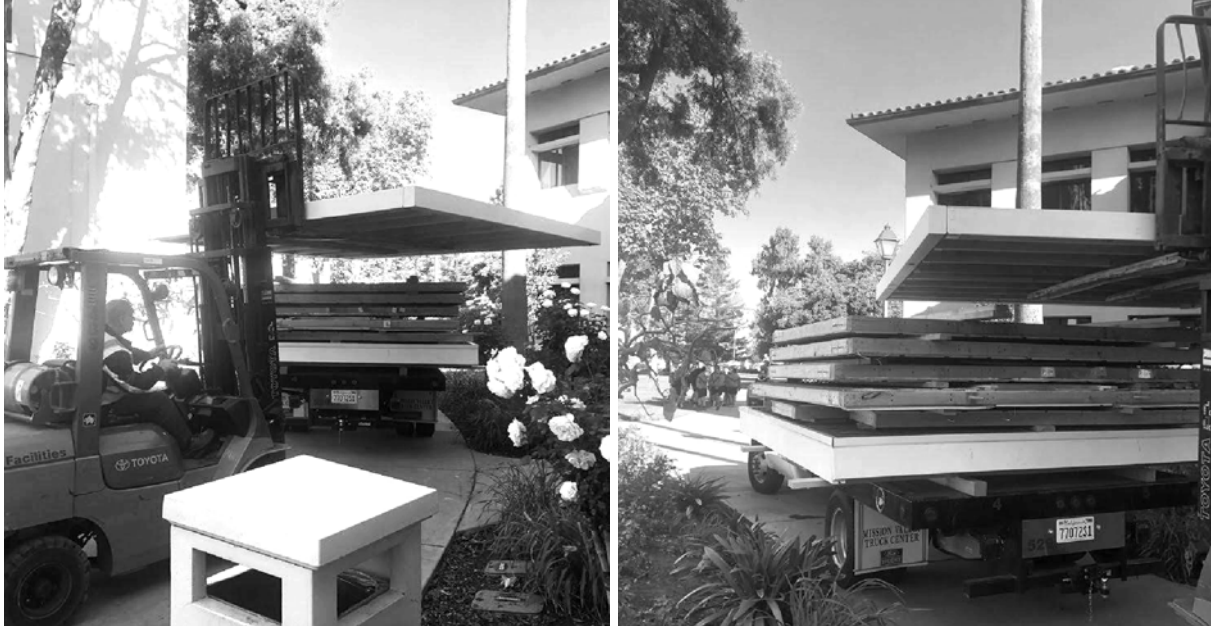
Figure H.19 - The floor was removed and stacked on the truck, concluding the dismantling procedure.
