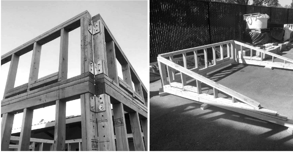
Figure H.6 - The height extensions were installed to ensure that they worked and then moved to the ground for roof construction.
