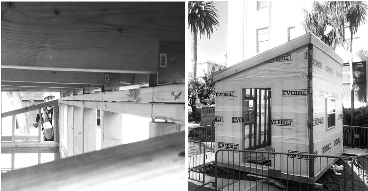
Figure H.10 - The roof was transported to the site and placed on top of the cabin.
