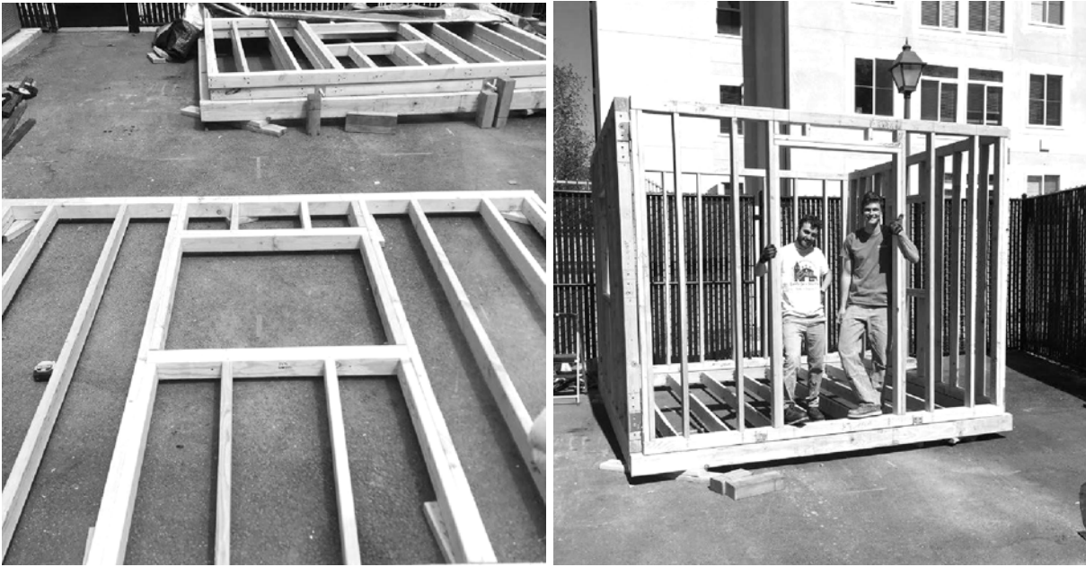
Figure H.4 - The walls were framed (left) and then erected to test the wall-to-wall corner connections (right).
