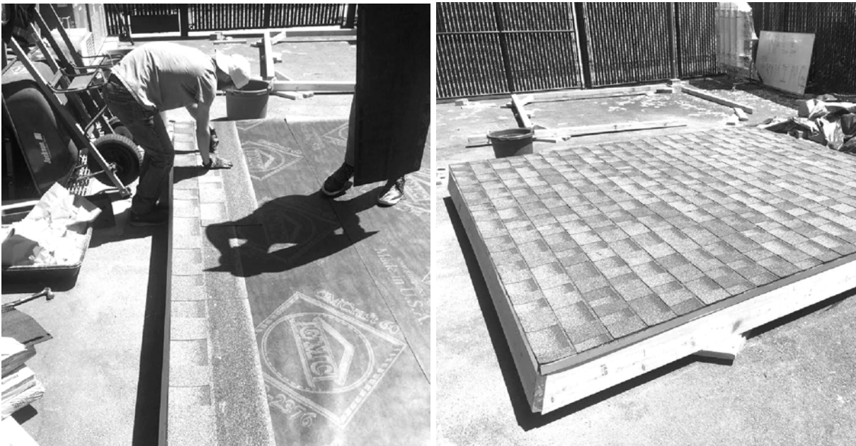
Figure H.8 - The roof was finished with roofing paper, flashing, and shingles on the ground.
