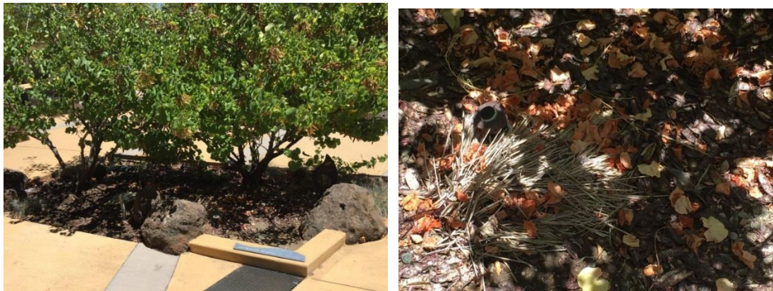
Figure 39. Campus Site 13 (2012) with an infiltration rate of 5.5 in/hr., and a total criteria score of 23 (Photo by author).
