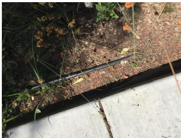
Figure 15. Exposed drip irrigation pipe at Municipal Site 21 (Infiltration Rate: 18.2 in/hr.) (Photo by author).
