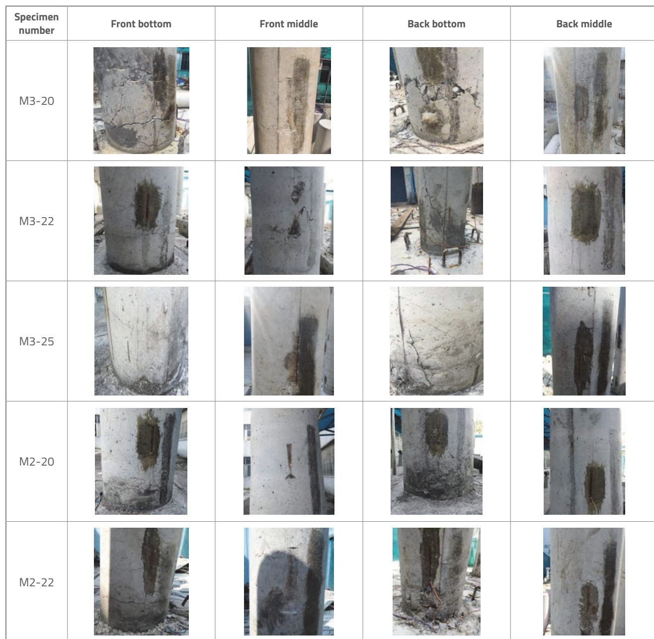
Figure 21. Specimen cracking pattern
