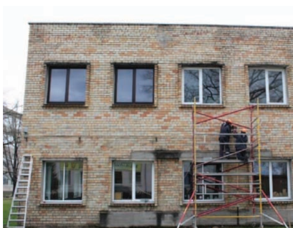
Figure 1. The façade in question, note the window casings, reinforced concrete elements and gas line.
