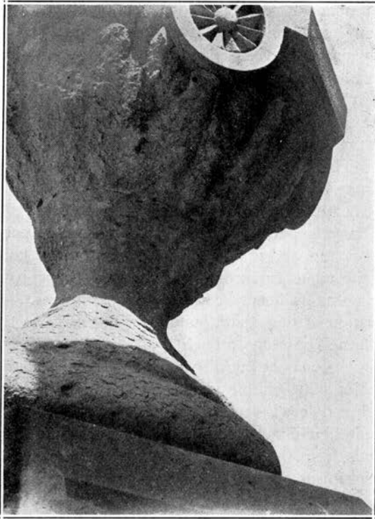
Fig. 5. View from below, of south side of urn at northwest corner of southeast dome, showing decay of blue stone in an apparently sheltered position.
