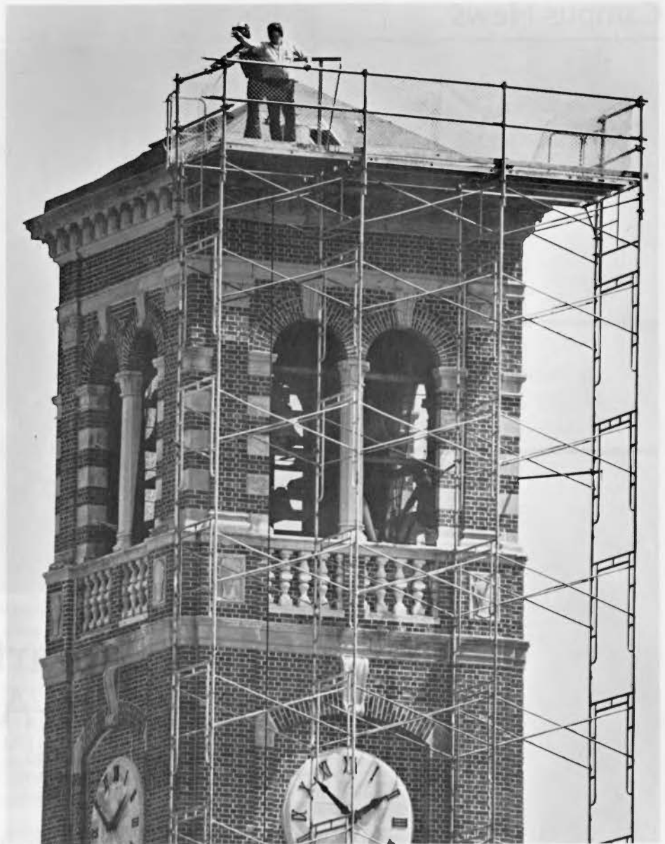
Maintenance and repairs to the Campanile this summer included replacement of the roof and other work. The campus landmark was shrouded in scaffolding for more than a month. Renovation of the carillon, the bell-playing instrument inside the Campanile, began in September and is still under way.
