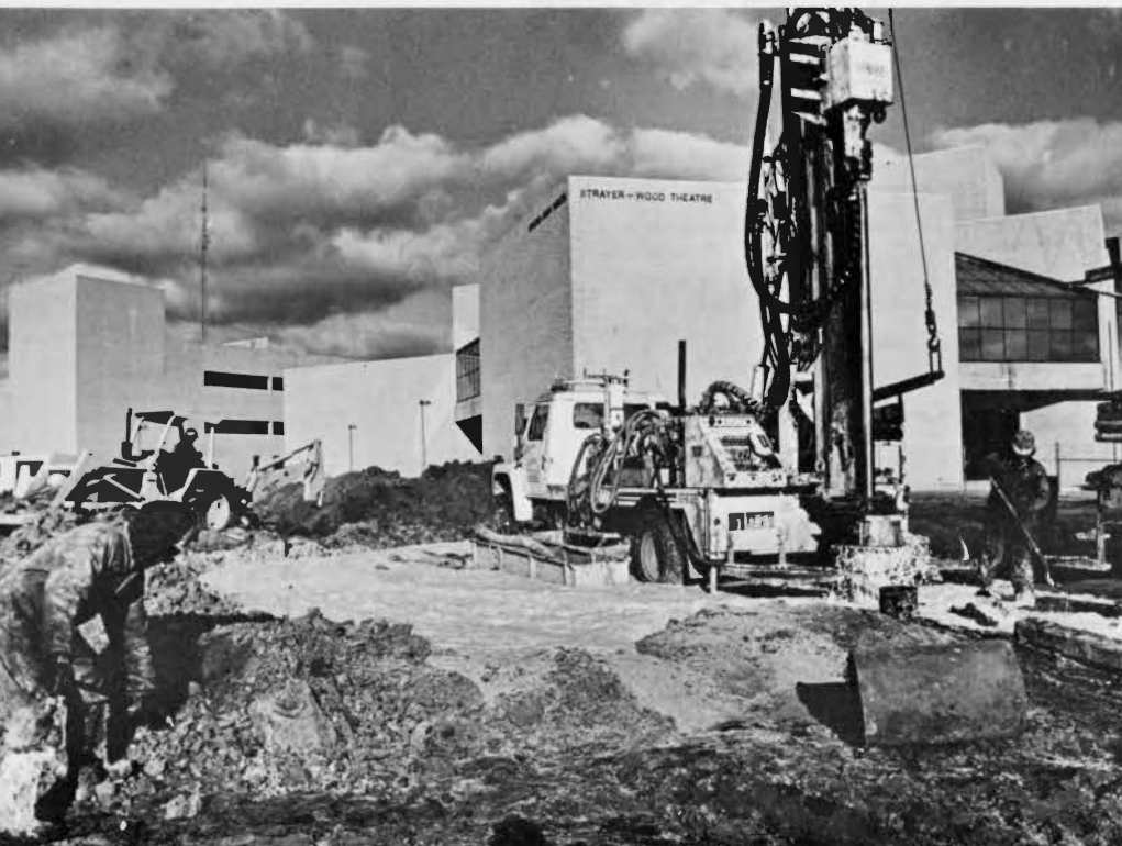
Construction of the second phase of the CAC building has resumed. Completion is scheduled for 1985.
