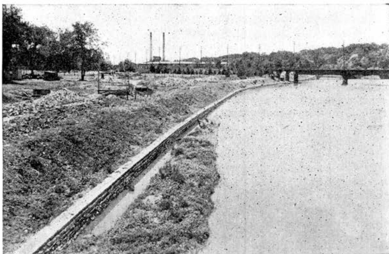
Fig. 4. Downstream view showing east bank of the Iowa River at Iowa City, Iowa. The stone wall was constructed first and then the unsightly material in the river (foreground) was dredged. The Iowa Avenue Bridge is the second bridge in the background. 1935.
