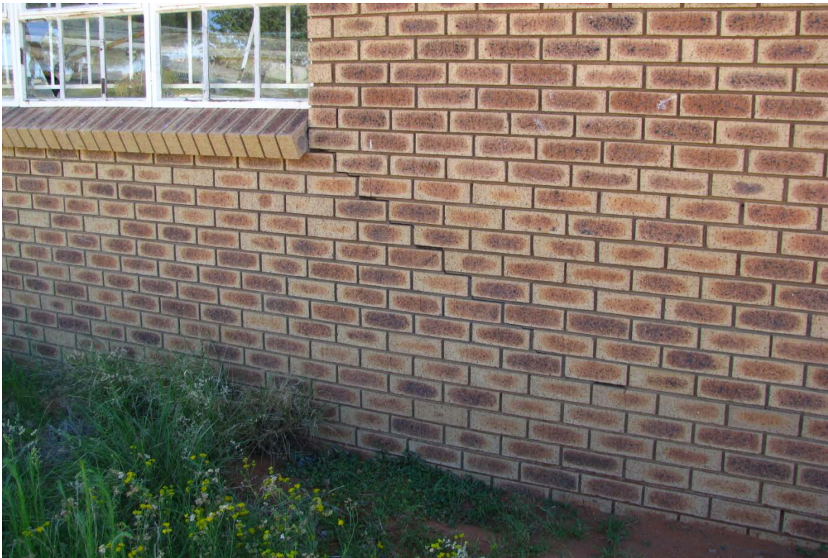
Figure F.4: Diagonal cracking below the windowsill, note the lack of a concrete apron slab (photo by author)
