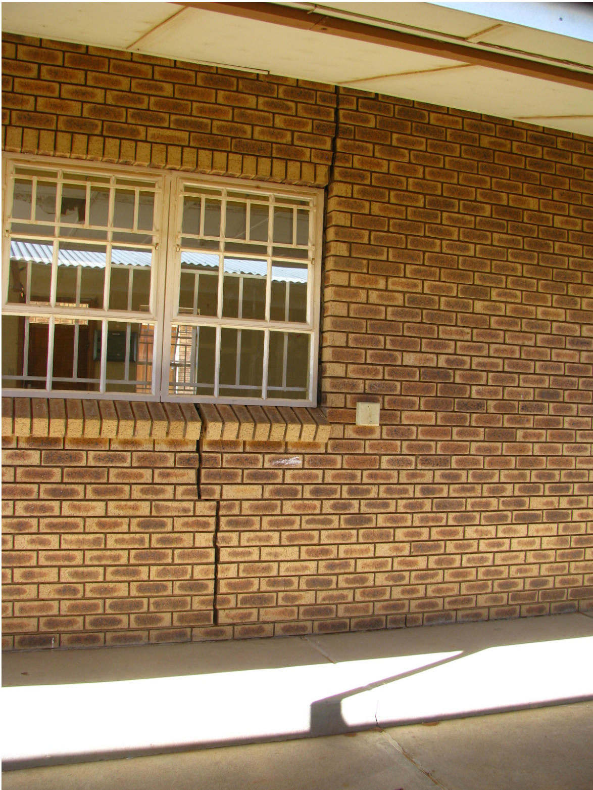
Figure F.3: Expansive cracking visible on the side of one of the current classrooms (photo by author)
