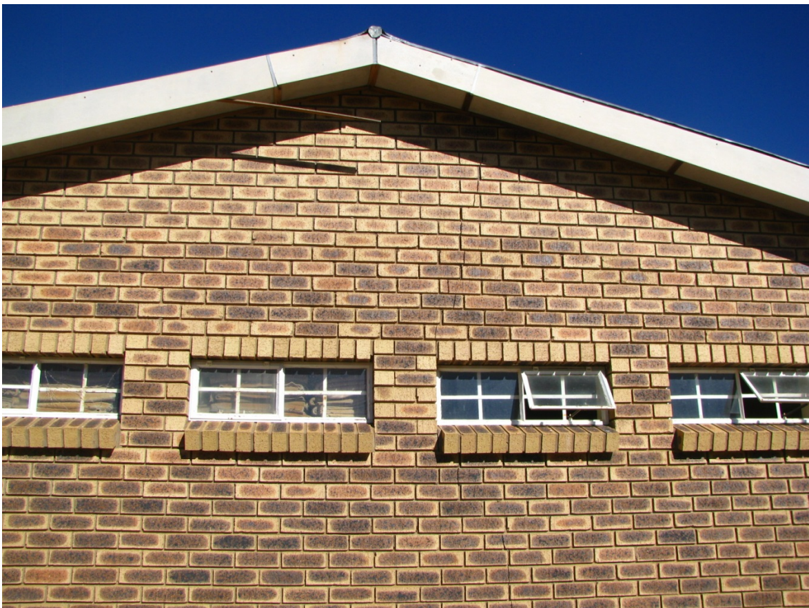
Figure F.5: Cracking near the roof of the class room (photo by author)
