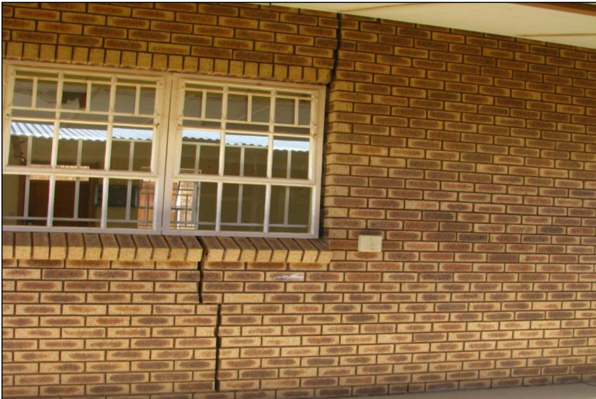
Figure 3.4: Expansive failure at a primary school in Luckhoff (taken by author, October 2014)
