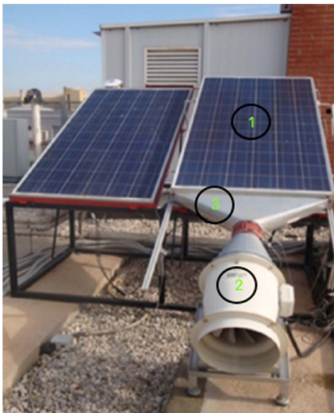
Fig. 10. Hybrid solar Photovoltaic/Thermal system cooled by forced air circulation [26].
