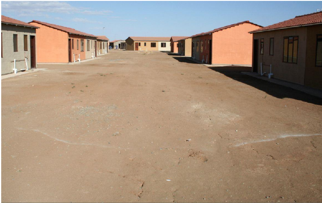
Figure 1.8: Shrinkage cracks at the ground surface.
