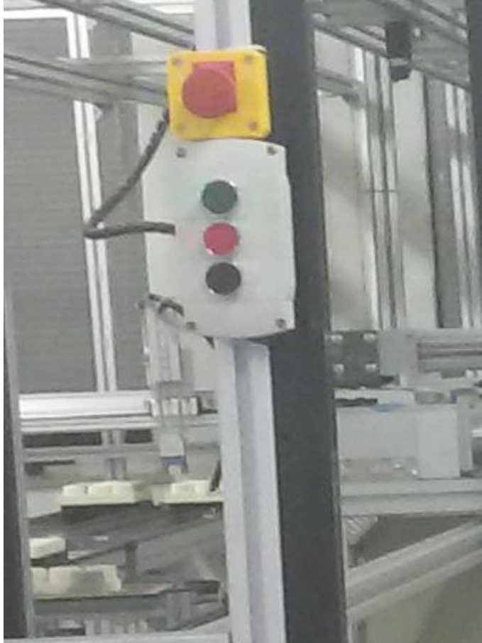
Figure 4.21: System control panel
