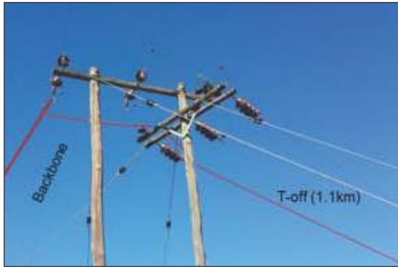
Figure 1: Photo of the pole where the contact incident took place
