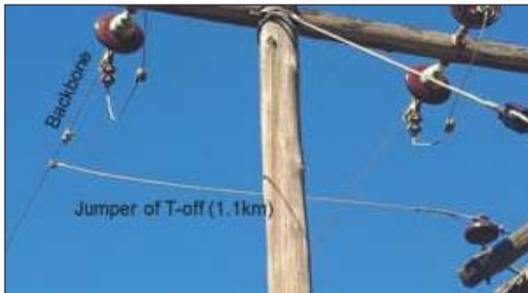
Figure 2: location where operator experience electrical shock
